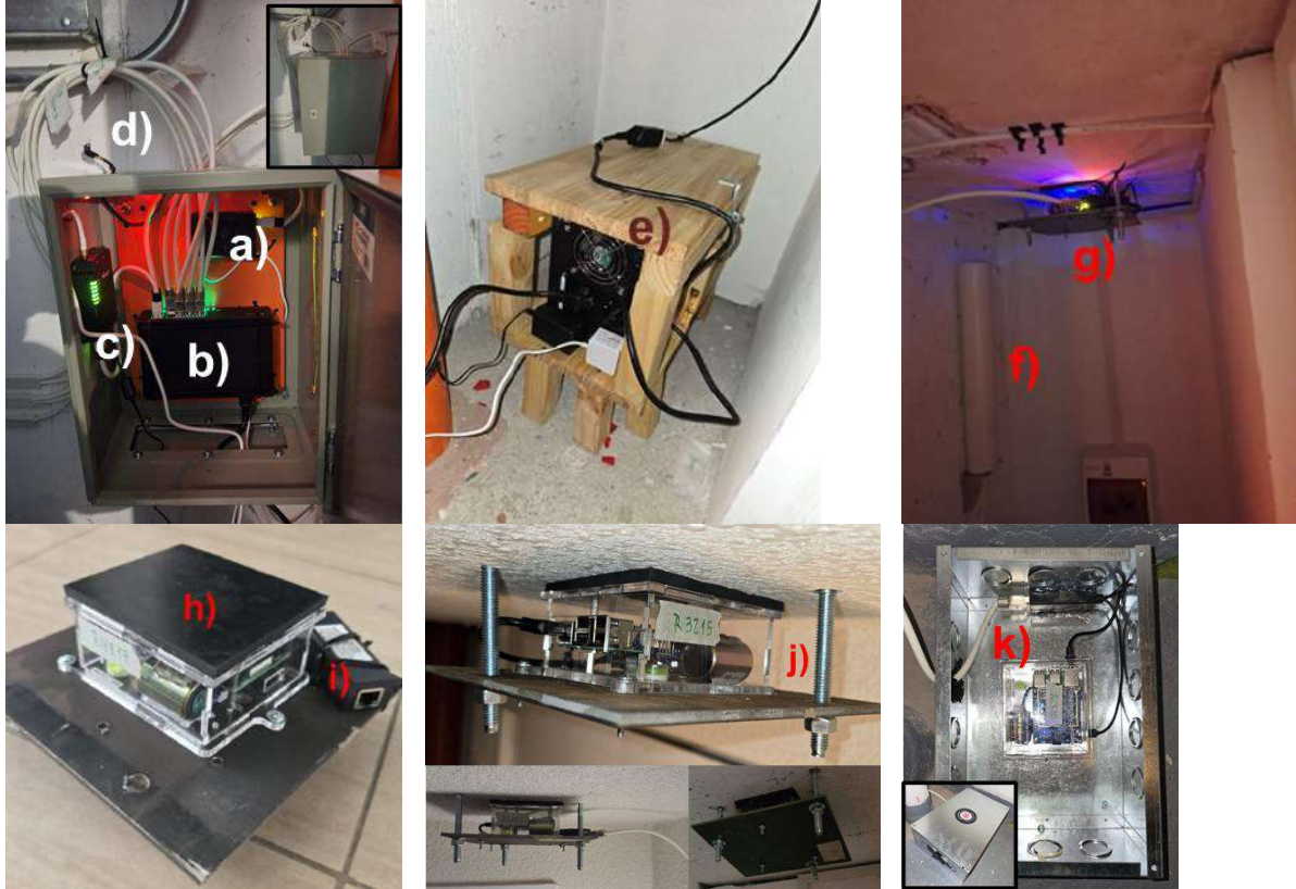
Figure 3. Photographs of equipment installation, a) RPi4B central, b) PoE Switch Milesight MS S0208-G , c) Router 4G Milesight UR32L-L04AU, d) BME 280 barometric sensor, e) UPS Hikvision 3000 VA / 1800 W , f) 4G Antenna (18dBi), g) RS4D installed on the roof, h) RS4D before roof's installation, i) JT-COM PoE splitter, j) details of RS4D roof's installation, k) RS4D installed on the ground floor.
